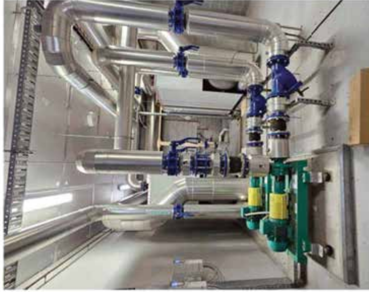
Figure 9 Installed primary-only pumping arrangement – primary heating pumps 1 & 2.
