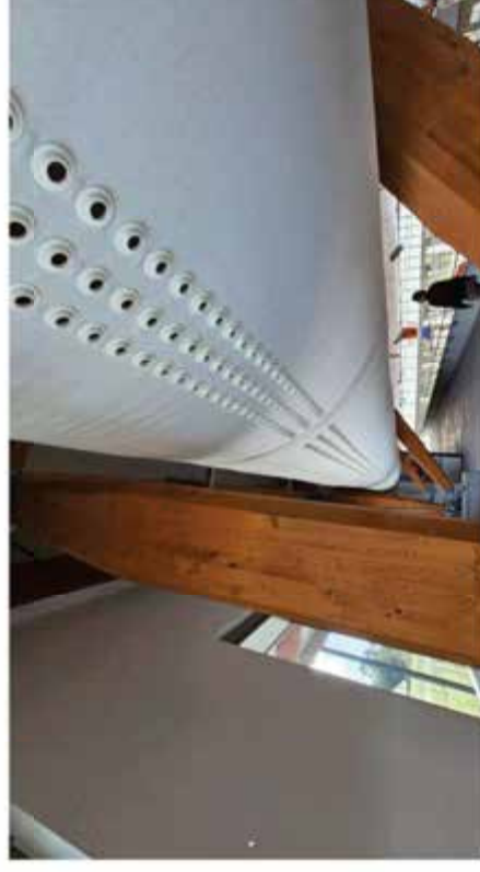
Figure 11 Fabric duct with jet nozzles.
