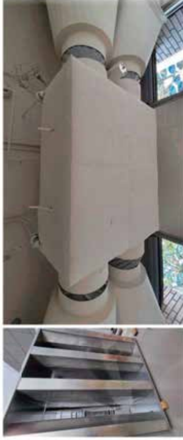
Figure 28 Typical air handling unit attenuator (left) and acoustic wrapping of ceiling hung ERV unit.
