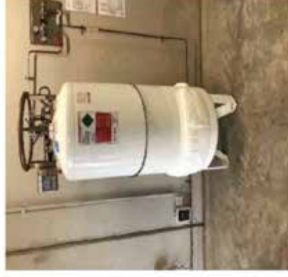
Photo 5: Internal location of CO2 Cylinder.
