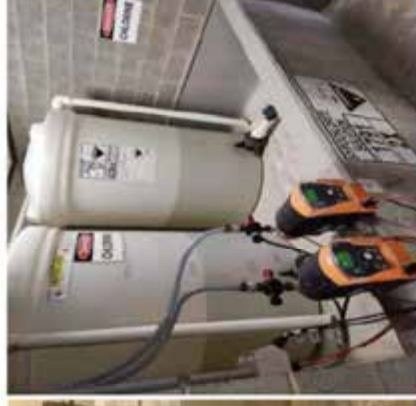
Photo 6: Current Chlorine tank and internal bund.
