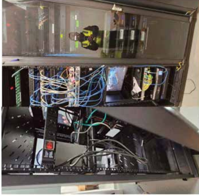
Figure 34 Existing Comms data rack
