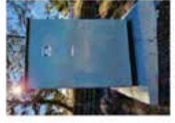
PHOTO: ELECTRICAL CABINET
