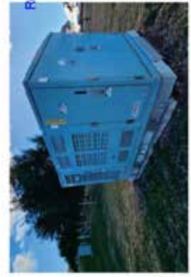
PHOTO: ELECTRICAL CABINET
