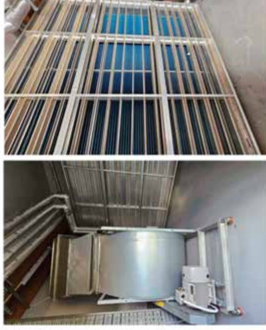
Figure 10 Supply air fan, heating coil with motorised damper within custom built air handling plant room.
