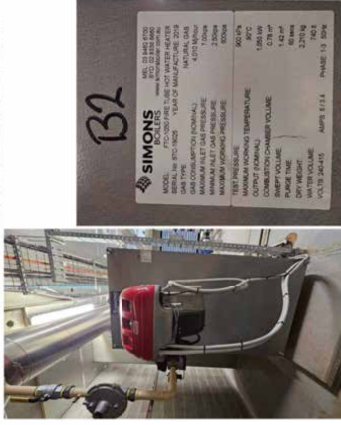
Figure 8 Installed condensing Boiler #2 by Simons Boilers.
