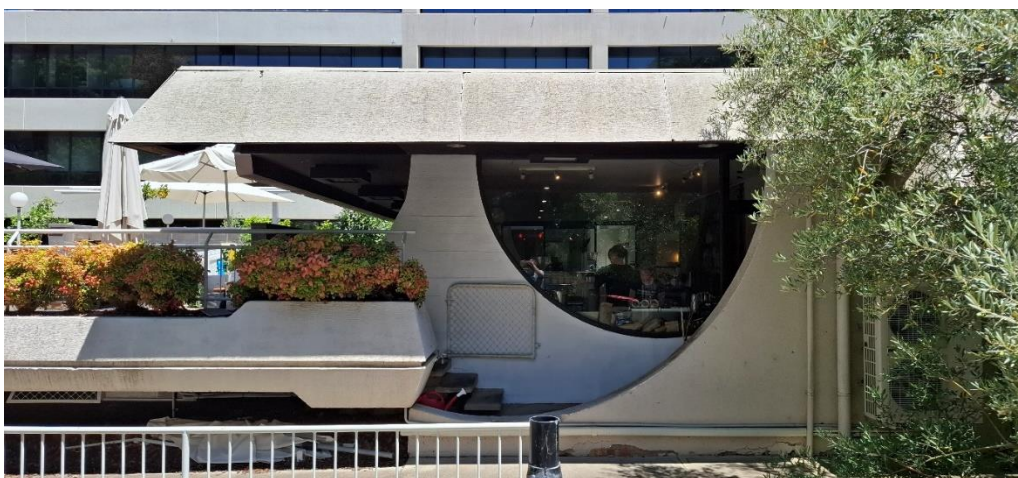
Figure 6 East end concrete features painted of rendered, PVC drainage and fibrous cement sheeting fascias (2026)
