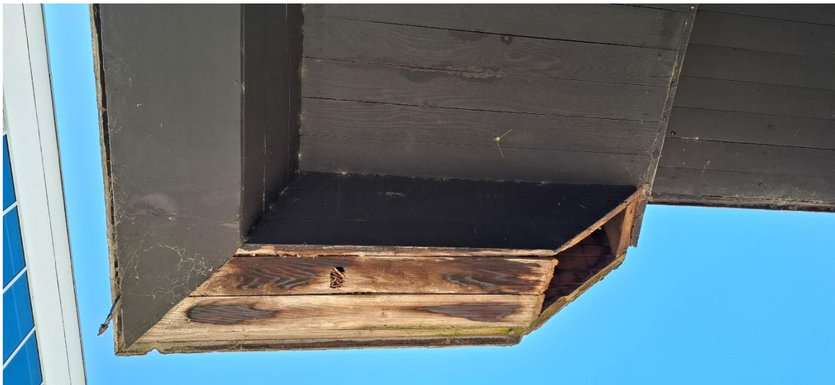
Figure 16 Some original material from the fascias may remain under the later cladding, but appears to be in poor condition (2026)
