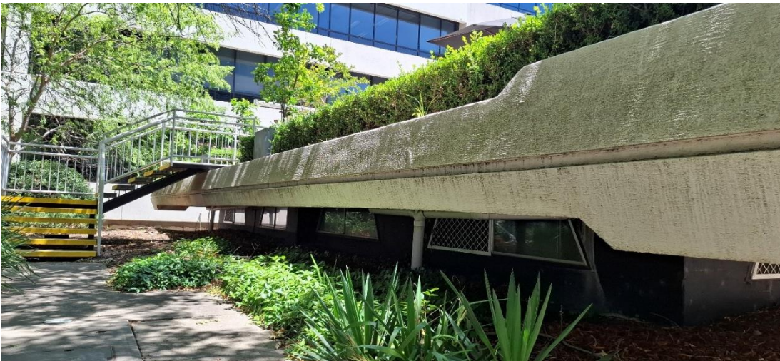
Figure 12 Later stairs, rendered finish and PVC pipe drainage (2026)
