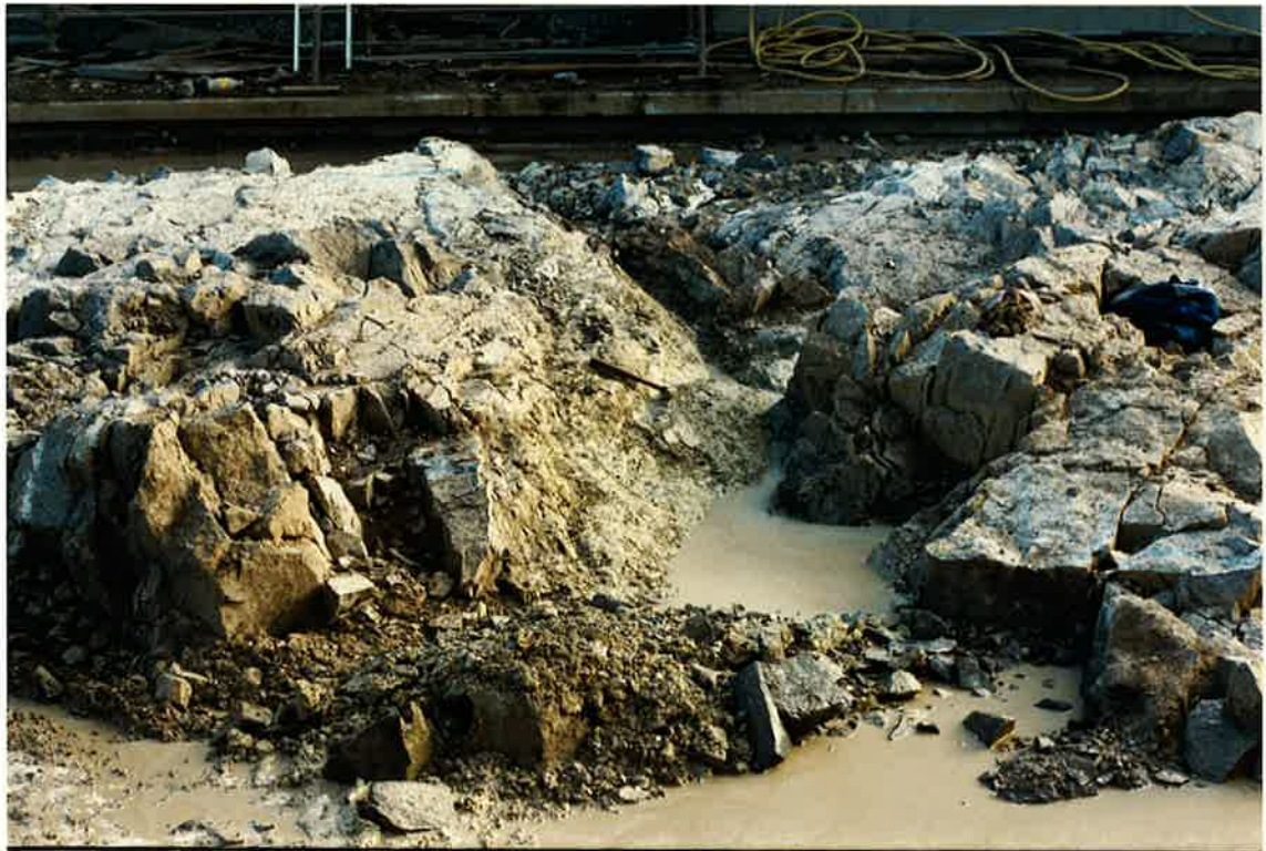
PHOTOGRAPH 15 Central Channel, west side, clean up of clay seam across site. July, 1987
