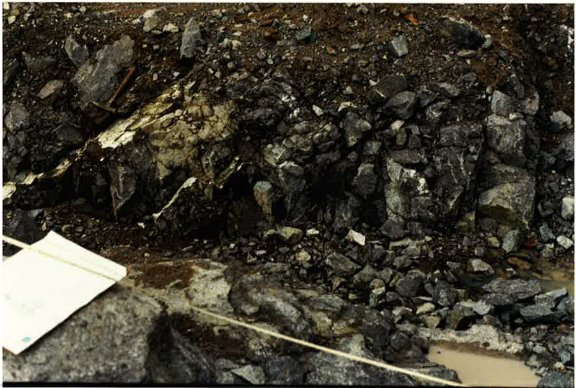
PHOTOGRAPH 11 Central Channel, closely jointed zones in foundation area. February, 1987
