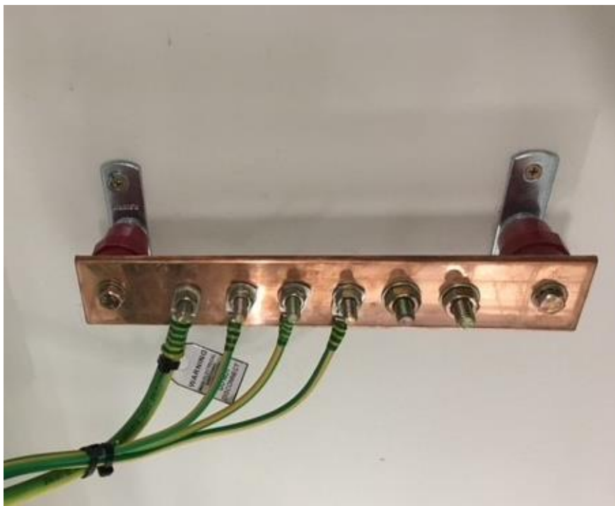
Figure 1: Comms Room Copper Earthing Strip
