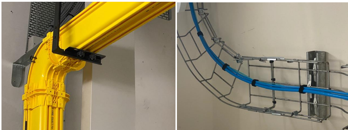
Figure 2: Example of yellow fibre duct and basket entering a Building Distributer cabinet A
