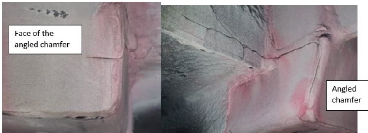
Figure 5: Cracks in L brackets visible after removal of bogie and protective coating (using dye penetrant test)
