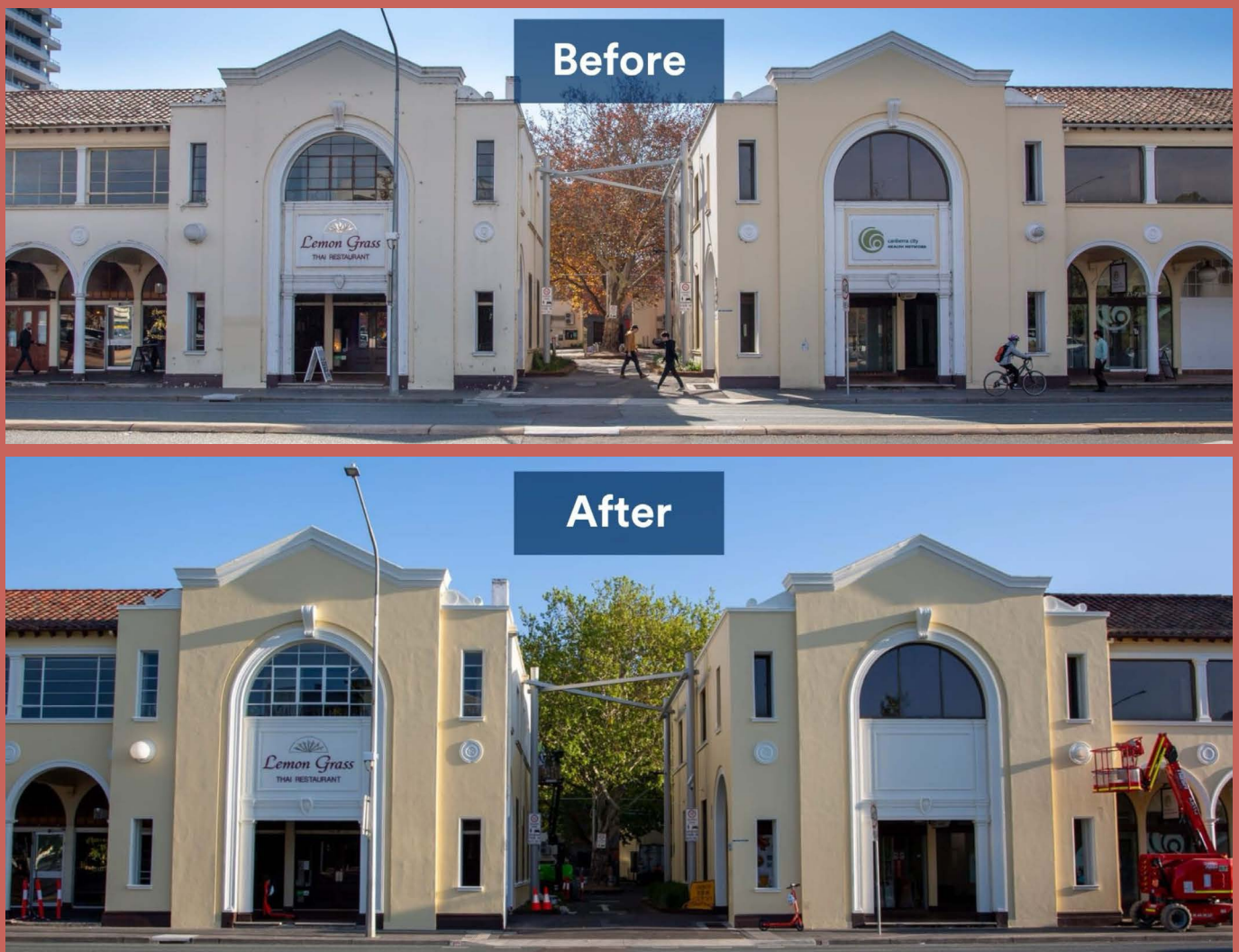
Figure 5 Melbourne Building at Odgers Lane entrance on London Circuit, before and after painting works
