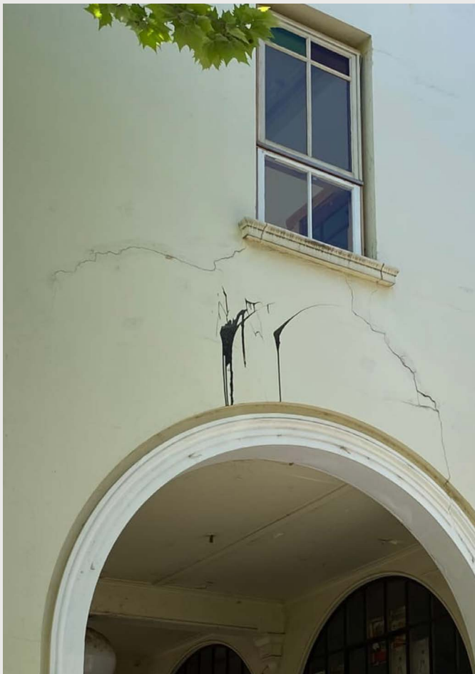
Figure 6 Cracked render on Melbourne building prior to painting works
