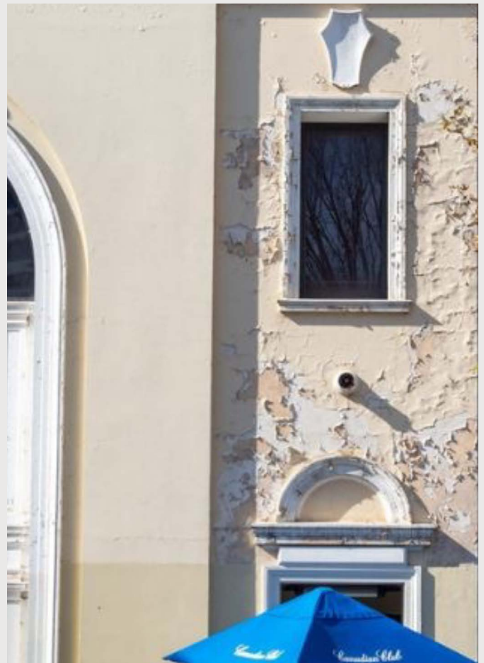
Figure 7 Peeling paint on Sydney building prior to painting works
