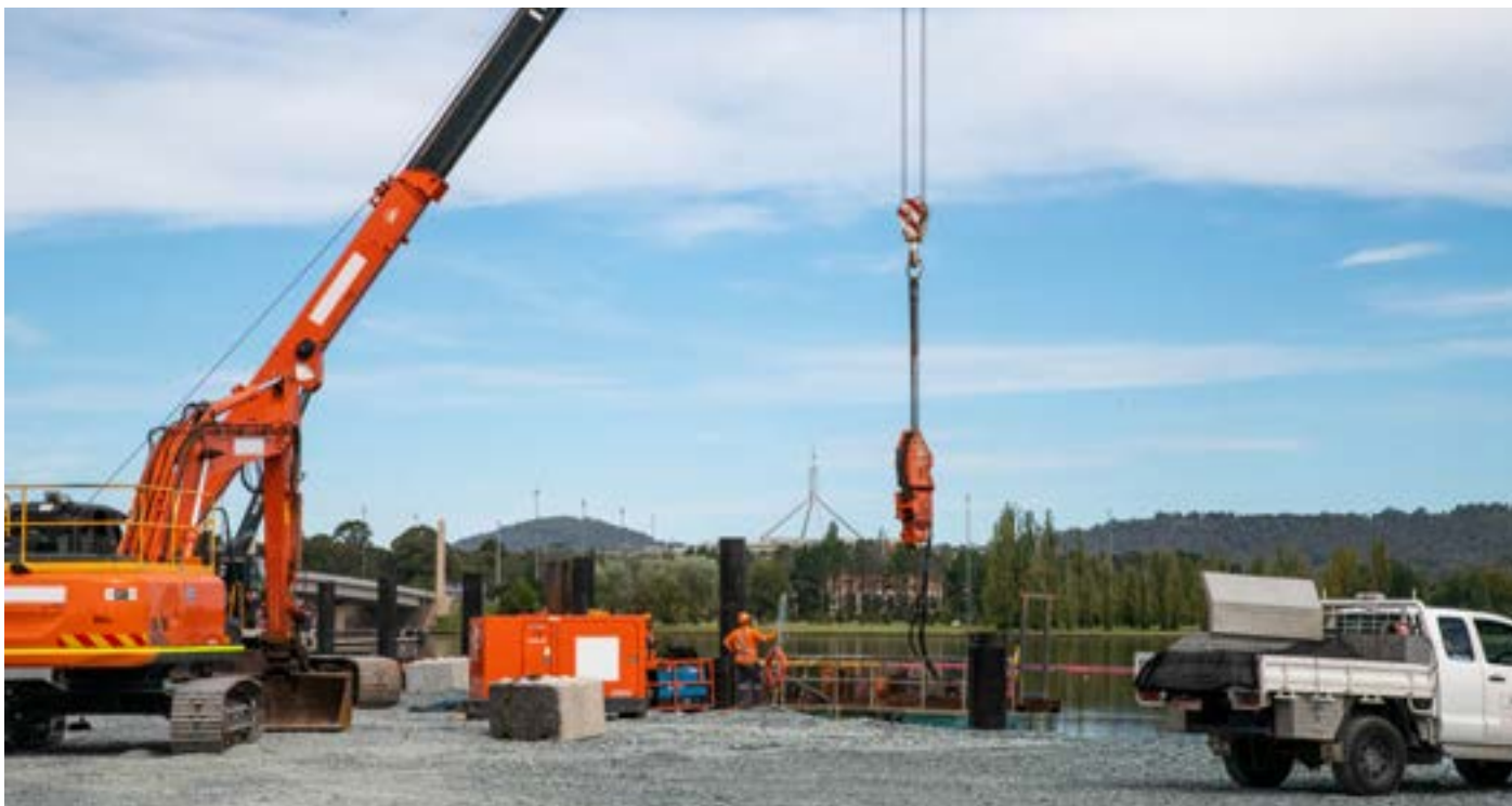
Construction team working on the extension of the boardwalk. Taken by Patrick Rose.
