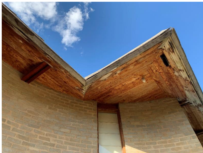
Figure 4: Soffits are water damaged and the fascias are buckling (ACT Heritage 2026).
