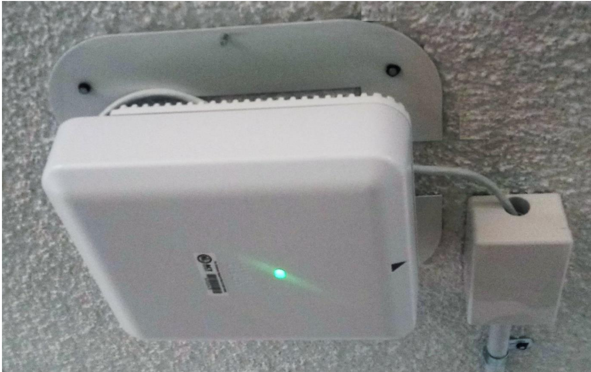
Figure 13 - Concrete Ceiling Mounted WAP
