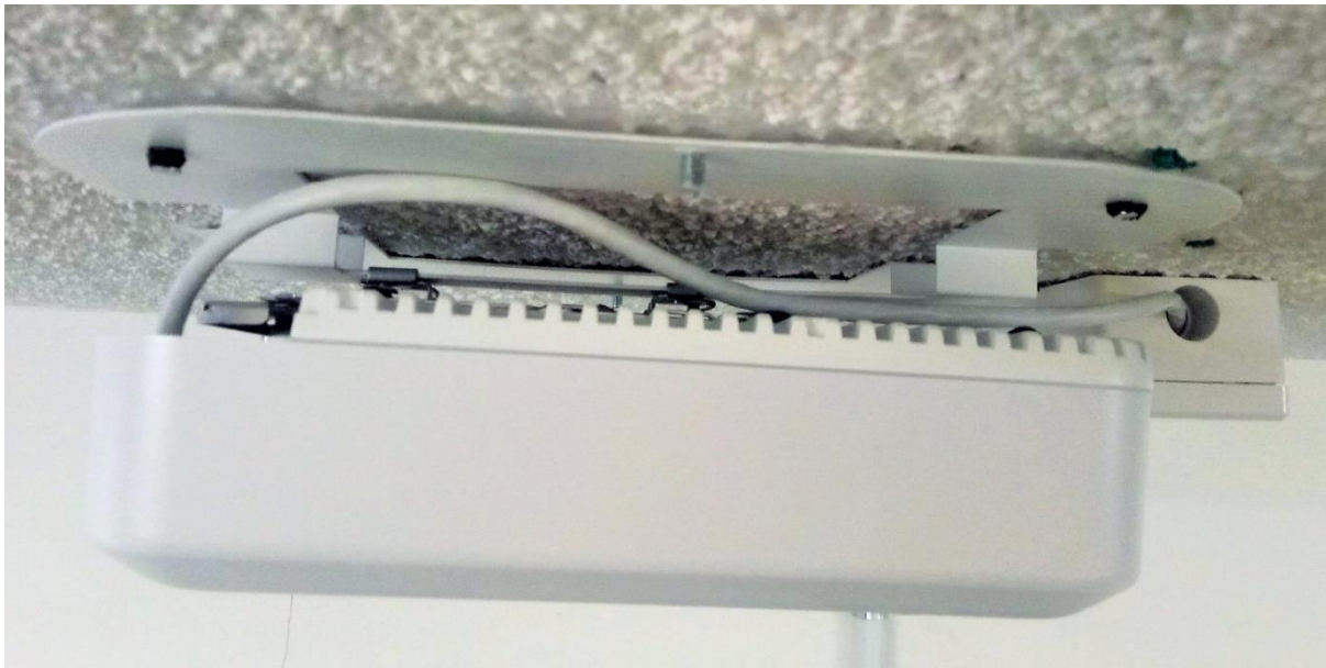
Figure 12 - Concrete Ceiling Fitting
