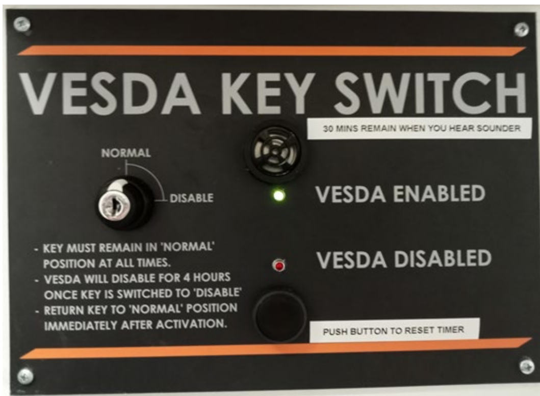
Figure 3 MASDS Isolation Switch
