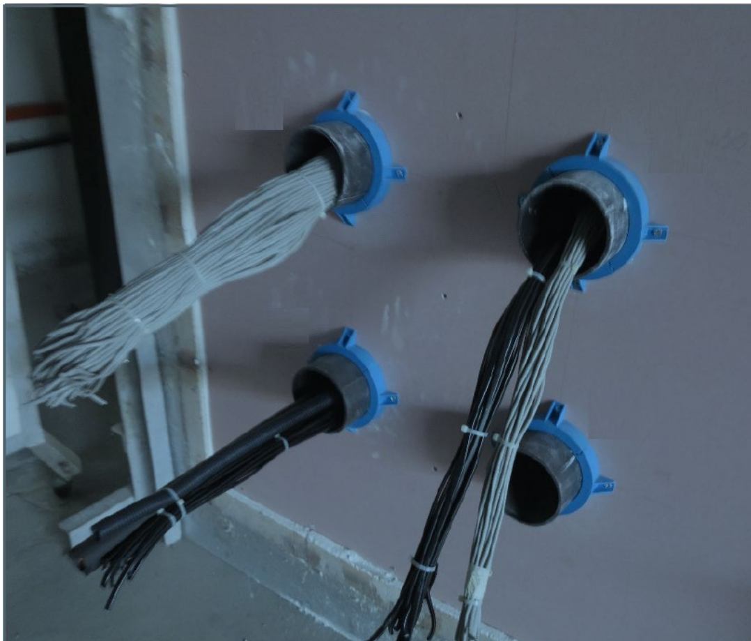
Figure 8 Example shows completed installation of Promastop® data, power and security cabling with spare for mechanical.
